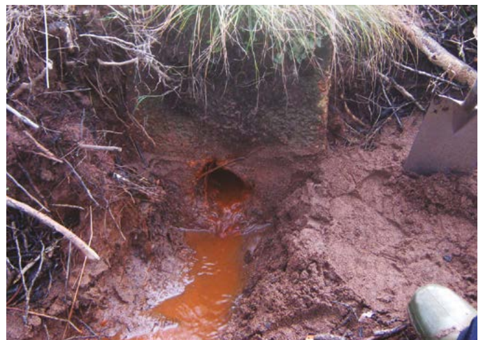
Figure 21. A blocked outfall can often be cleared in a matter of minutes with a spade
