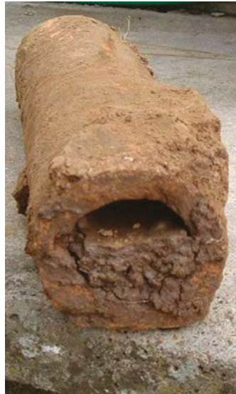
Figure 22. Silted clay drain
