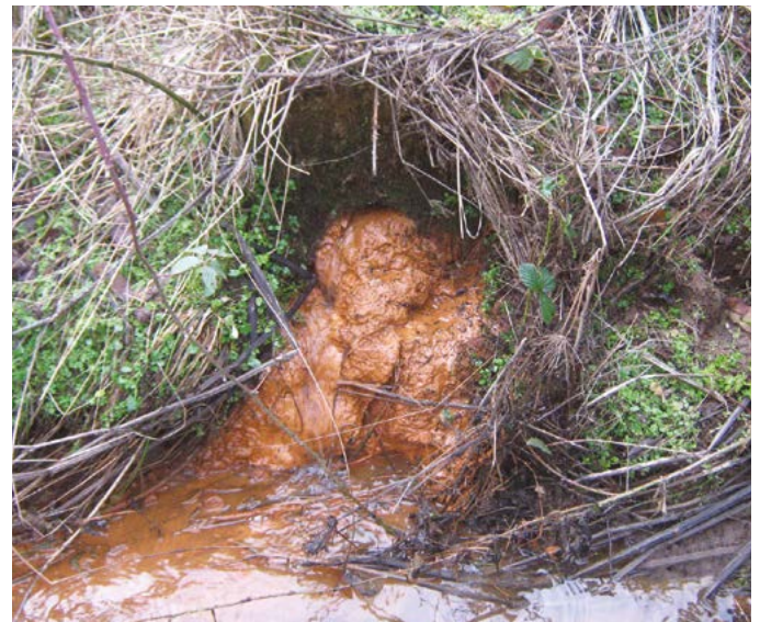
Figure 24. Drainage outfall blocked by ochre
