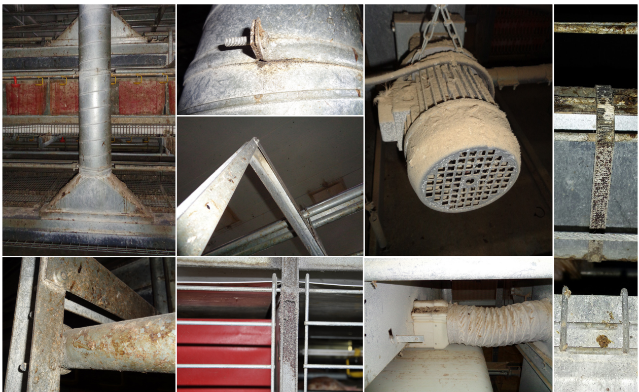
Figure 4: Examples of areas that require thorough cleaning such as manure belt aeration system, motors, tubing, joints, support structures, cable tie
