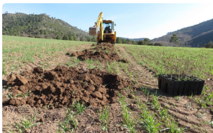
Figure 3. Soil preparation with a backhoe excavator in Can Pallot site. Author: AGS-CTFC | © CC BY 4.0
